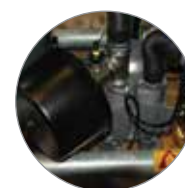
Inlet blower filters
