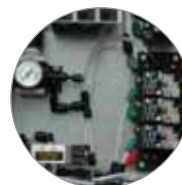
Pneumatic control systems
