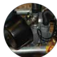
Blower inlet filter
