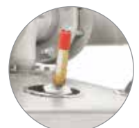
Vessel safety valves
