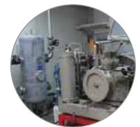
Pressure testing of components
